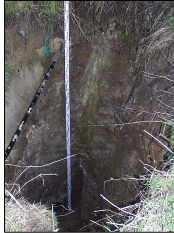
A cavity due to dissolution on A2 (Highways England)
