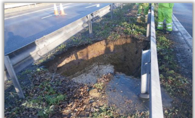
Subsidence sinkhole due to a dissolution feature in chalk, located on the M2
